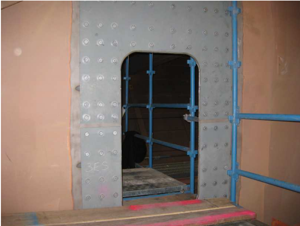
Enlarged Bulkhead entry doors replaced 'crawl holes' where possible, significantly improving people access
