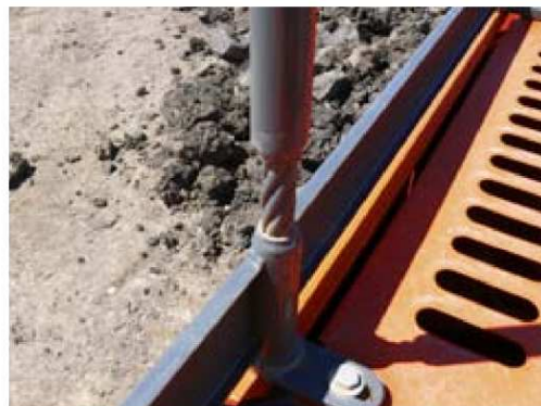
< Guardrails incorporating a section of wire rope to reduce fatigue cracking due to vibrations.
