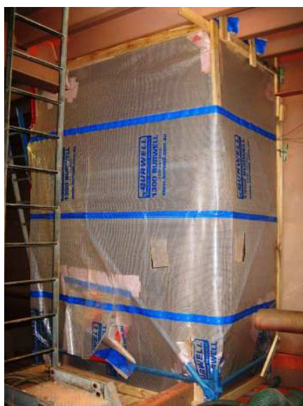
Paint removal areas were isolated close to the work to prevent the spread of paint dust
