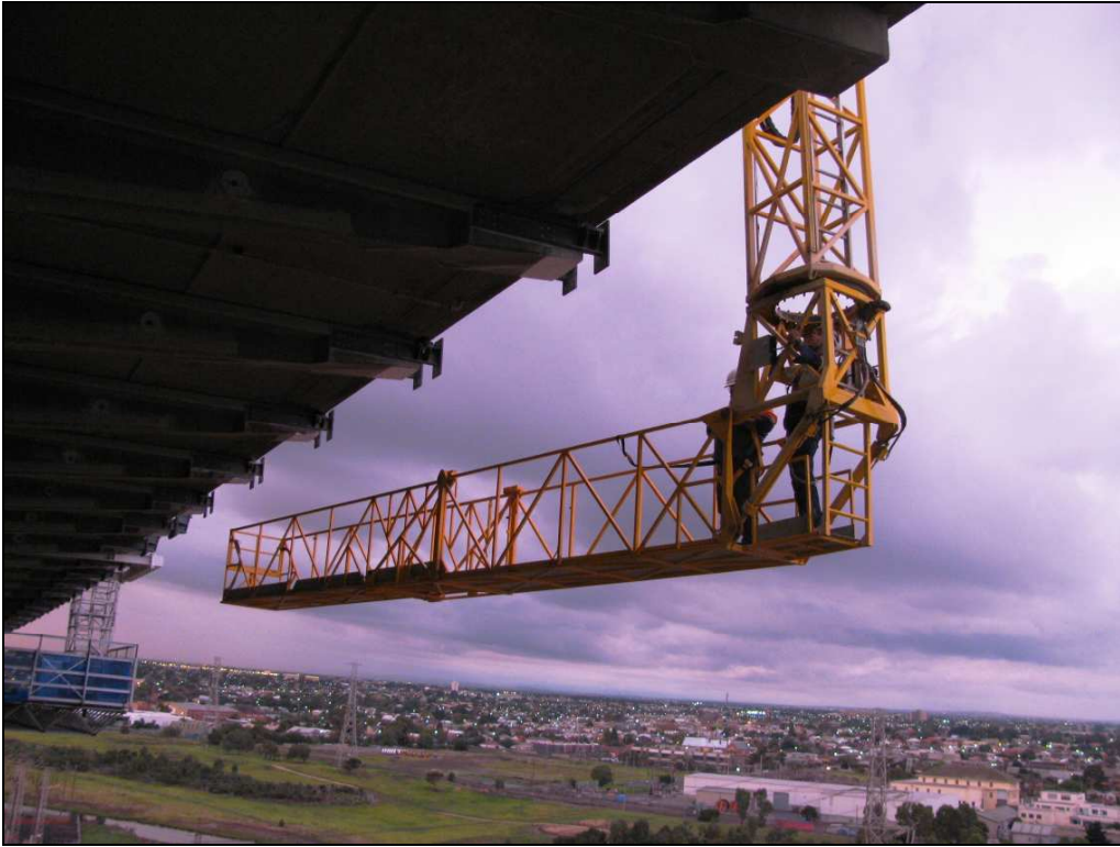
Lowered Boom of trial inspection unit being slewed into position under the bridge.
