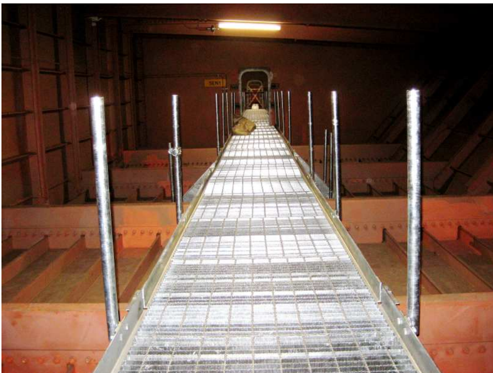
Modern standard walkways with guardrails and step access to invert of bridge under construction.
