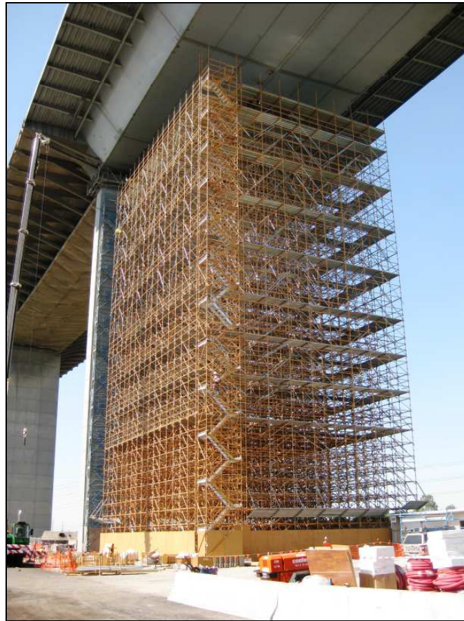
One of the largest bird cage scaffold structures. Two of these were installed to facilitate the placement of showers, change and lunch rooms close to but isolated from the work areas. This was necessary to contain the spread of the red lead paint dust.
