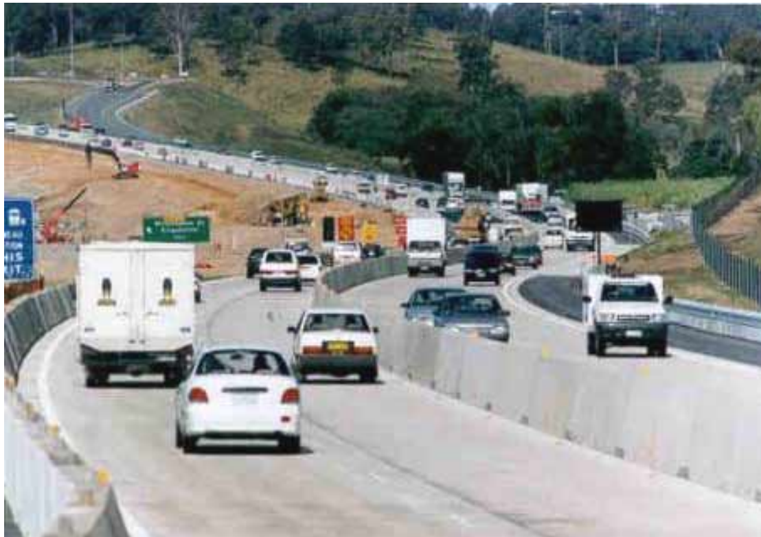
Figure 1 – Positive Separation by Concrete Barrier
